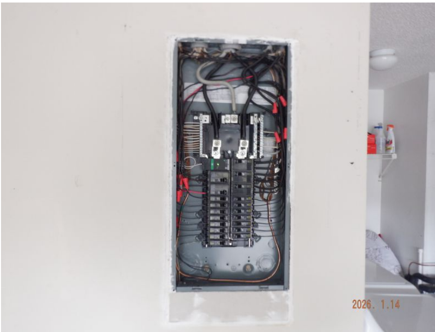
Interior Panel Wiring
