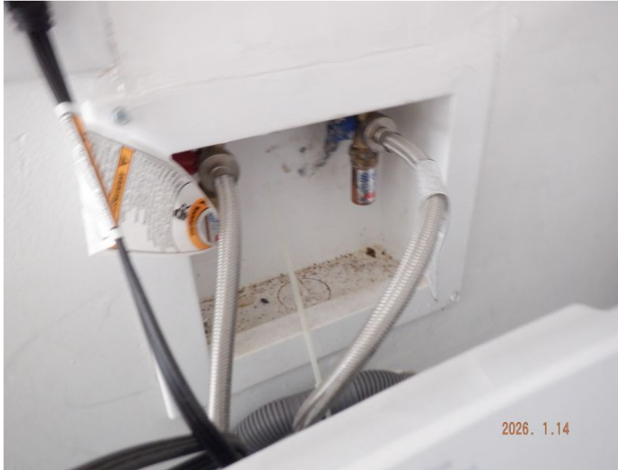
Washing Machine Plumbing
