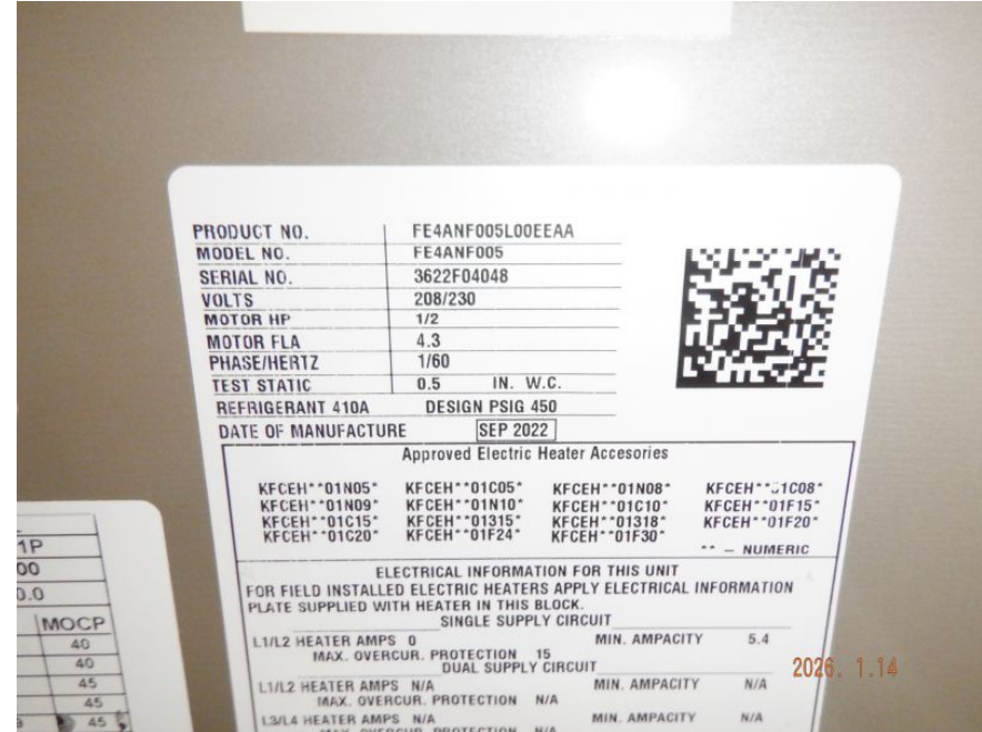
Air Handler Manufacturer Sticker/Plate
