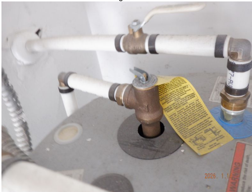
Water Heater Pressure Valve
