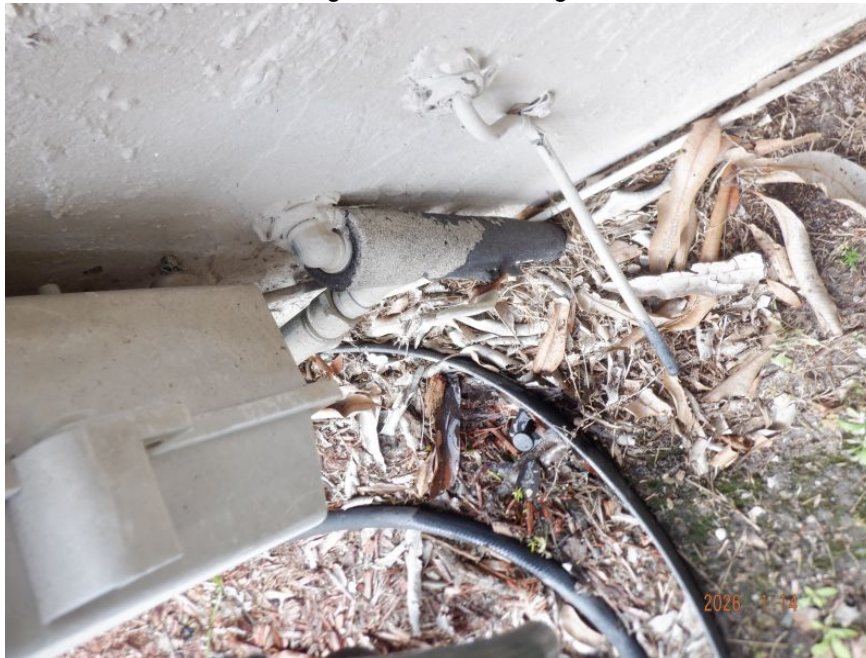
Main Supply Shut-Off Valve
