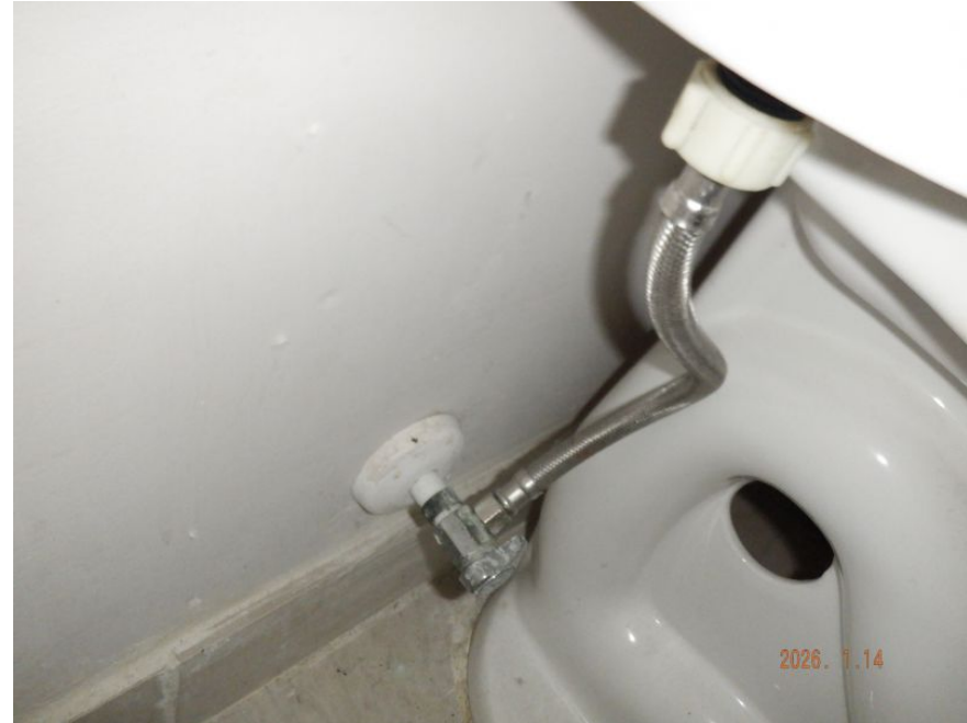
Toilet Shut-Off Valve
