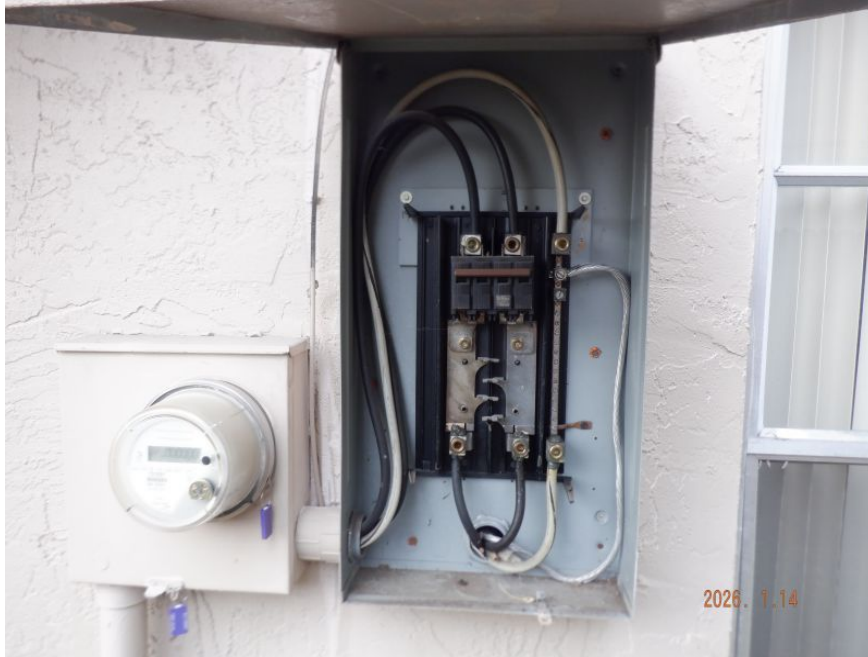
Exterior Panel Wiring
